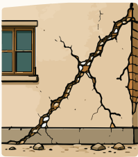
significant structural cracks
